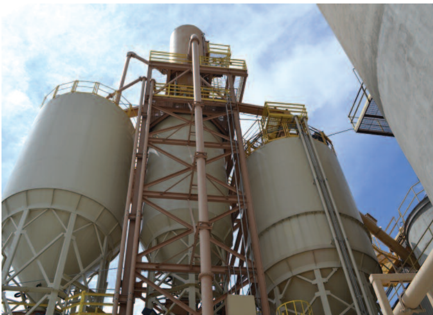
The blended cement products are conveyed from the pneumatic blending conveyor to one of the 200-ton-and-greater silos at the Omaha, Neb., facility.
