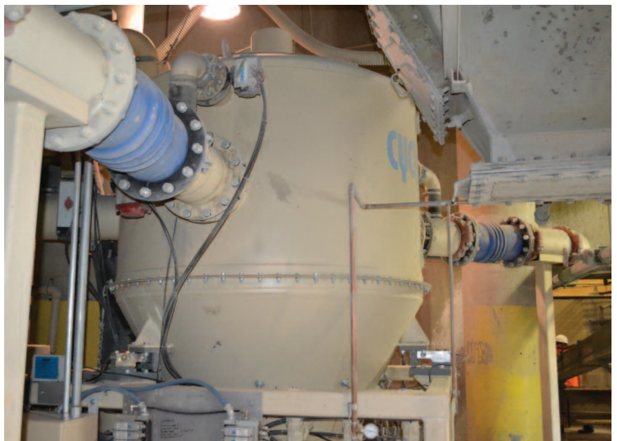
The CB Series pneumatic blending conveyor installed at Central Plains Cement allows the facility to weigh, batch, and blend up to five materials and convey the blend to loadout.
